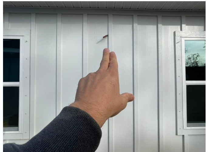
Siding damage location
