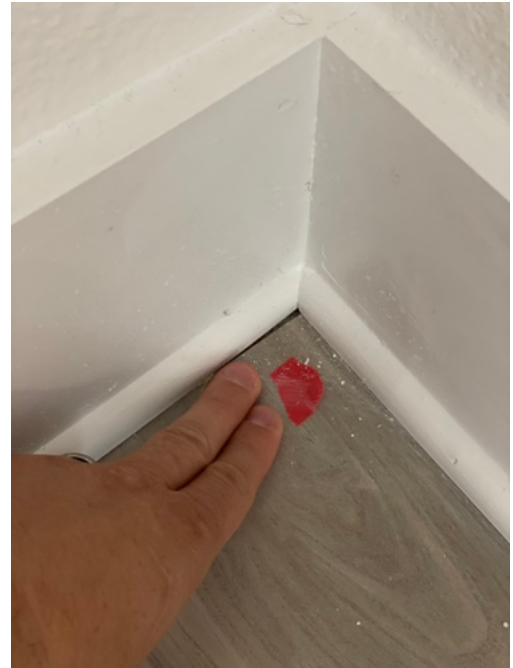
Gap between flooring and baseboard trim
