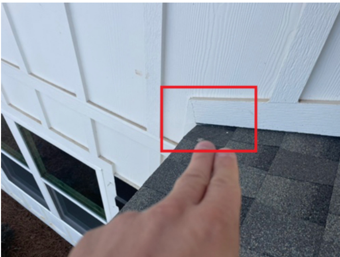
Missing diverter flashing
