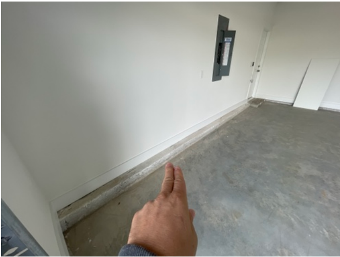
Garage foundation wall has cut J bolts where wall was moved.
