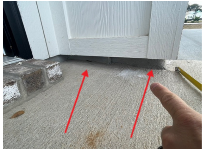
Bottom sill plate not properly sitting on foundation wall.
