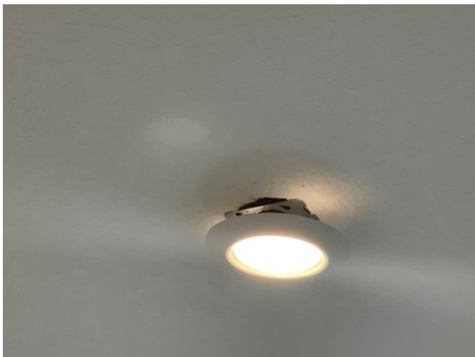
Loose LED light at front entrance hallway
