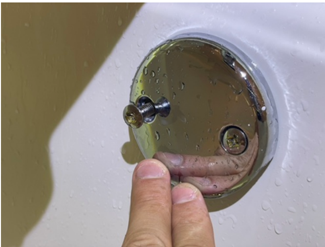
Loose overflow cover
