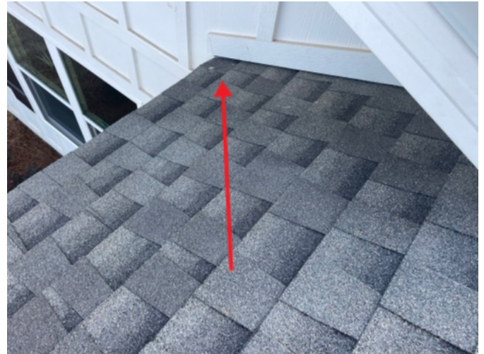
Location of missing diverter flashing.
