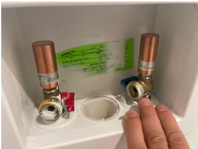
Twisted cold water valve
